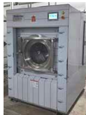
Washer-Extractor in Laundry
